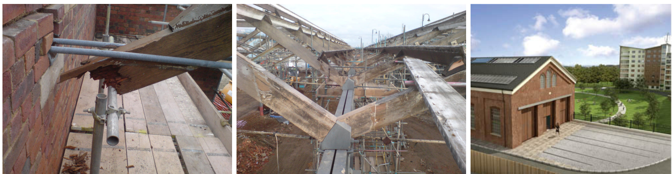
I-r: A decayed truss end, a series of repaired roof trusses and an artist's impression of The Royal
