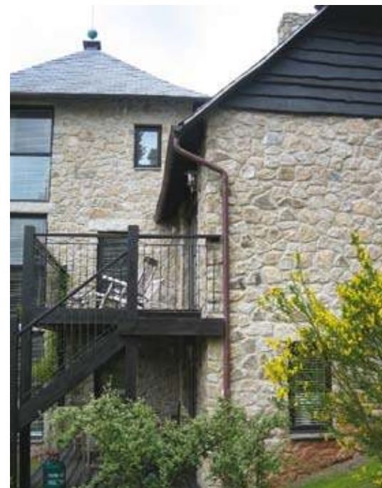
External view of property with high radon levels successfully remediated by ProTen Services
